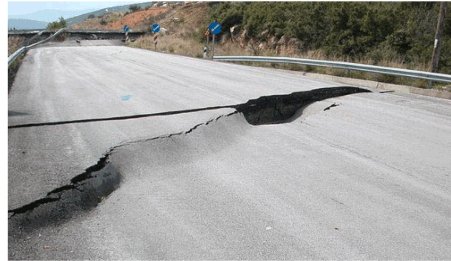
Fig. 1 Potential damage due to expansive soil
